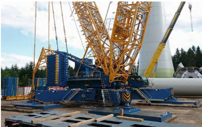
Figure 2: 650 ton Pedestal Crane
